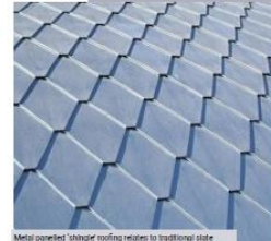
Metal panels 'shingle' roofing relates to traditional slate roofs, whilst using a more contemporary and dynamic material
