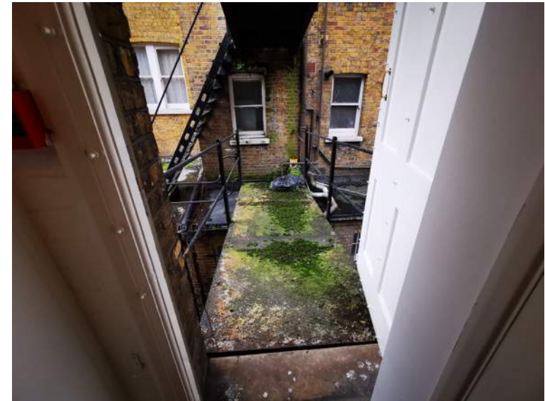
Fig. 21. dilapidated egress bridge poses safety risks
