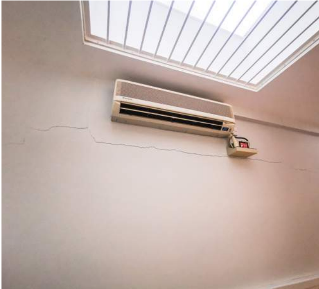
Fig. 30. horizontal crack on lower ground floor flank wall
