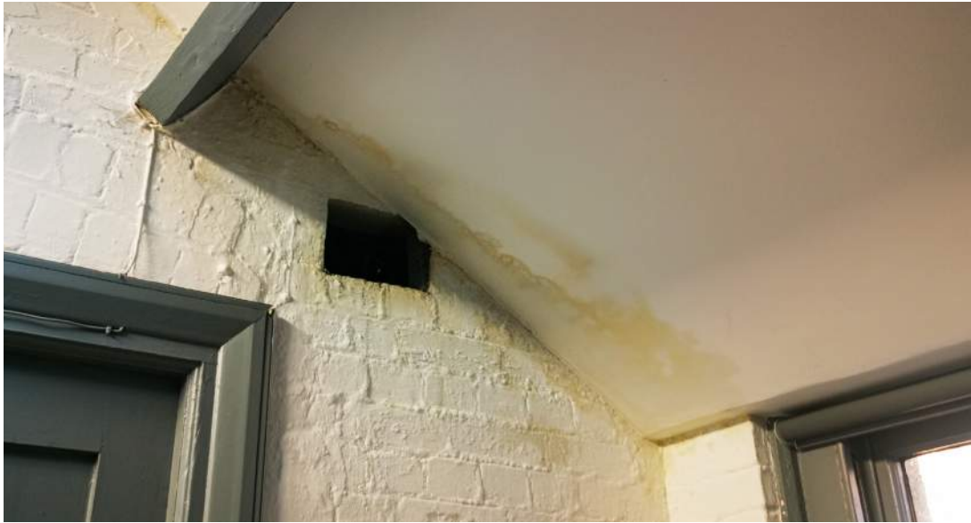
Fig. 27. water ingress inside roof, picture taken two weeks after fresh paint
