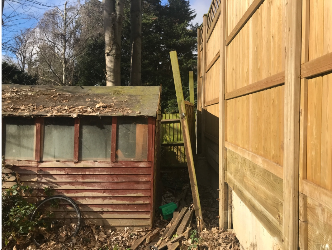
View of the existing garden shed and the side boundary with No. 22 Chesterford Gardens
