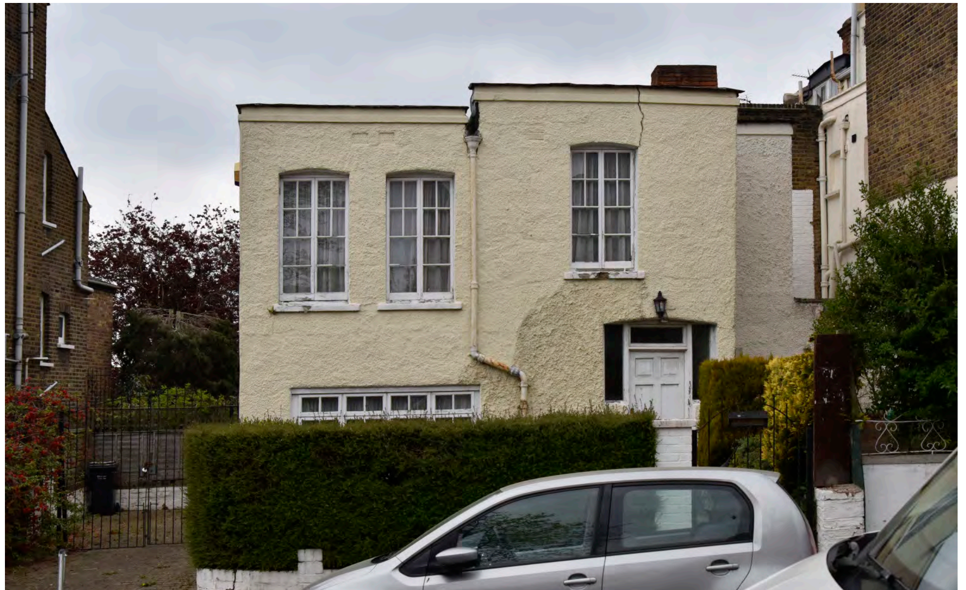
The Cottage seen from the street. The front facade shows clear signs of structural issues.
