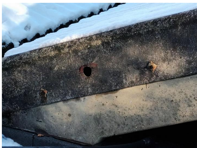
Figure 4: Feature C. Small hole in (asbestos?) roof, west facing (previously identified and still in the same condition)
