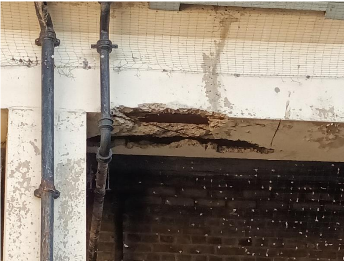
Figure 6: Feature E. Large cavity in roof, South facing, new feature
