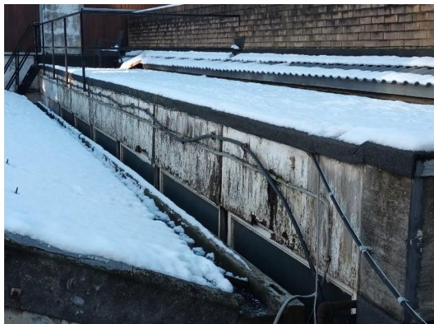
Figure 3: Feature B. Decayed wall cladding, West facing (previously identified and still in the same condition)
