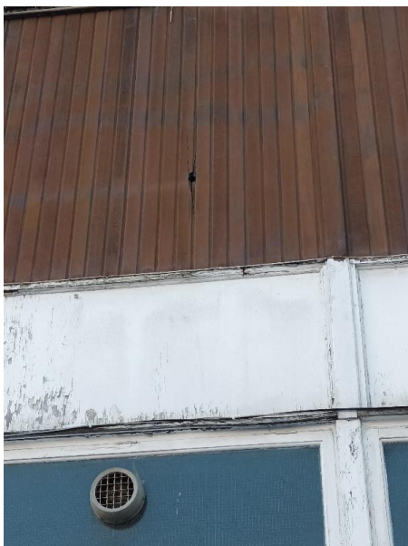
Figure 2: Feature A. Small hole in wooden paneling, north facing (previously identified and still in the same condition)
