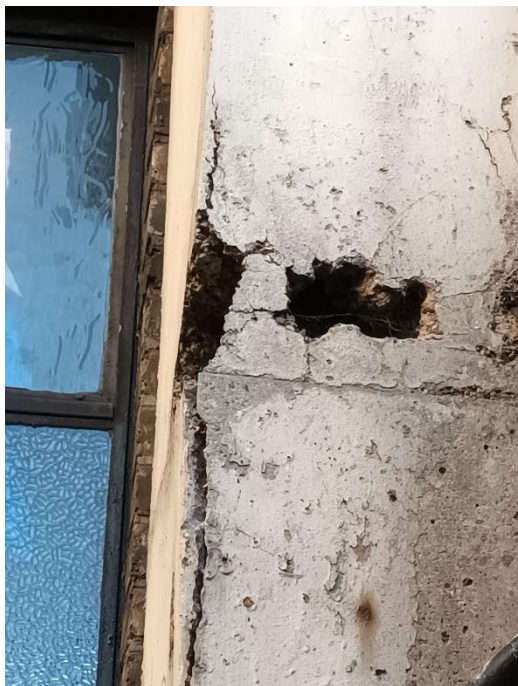
Figure 7: Feature F. Large cavity in wall, South facing, new feature
