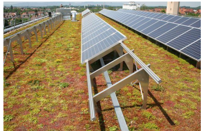
Figure 7: Monocrystalline PV arrays
