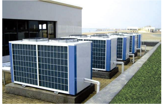
Figure 10: Outdoor units of ASHP
