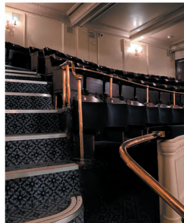
Uneven step risers in the upper circle
