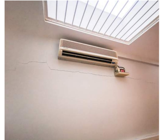
Fig. 30. horizontal crack on lower ground floor flank wall
