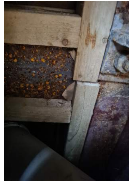
Fig. 29. surface rust on ground floor steel beams close to lower roof drainage
