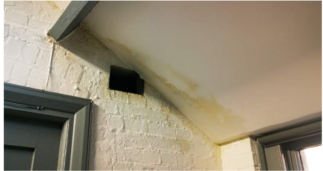
Fig. 27. water ingress inside roof, picture taken two weeks after fresh paint
