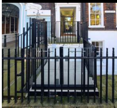
Lightwell lift - 1 New Square
