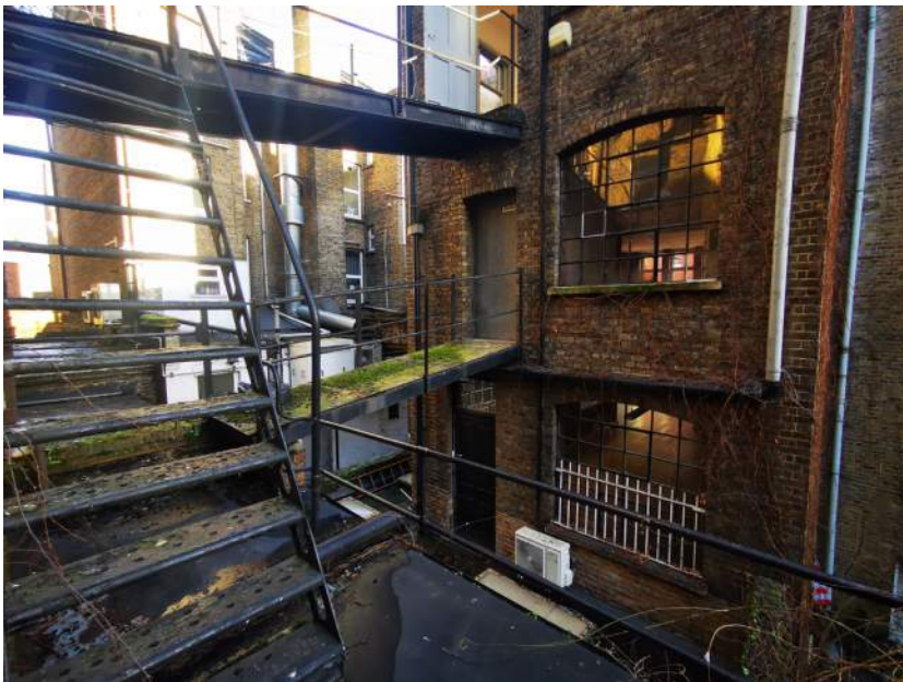
Fig. 28. dilapidated egress bridges pose dangers to occupants and neighbours
