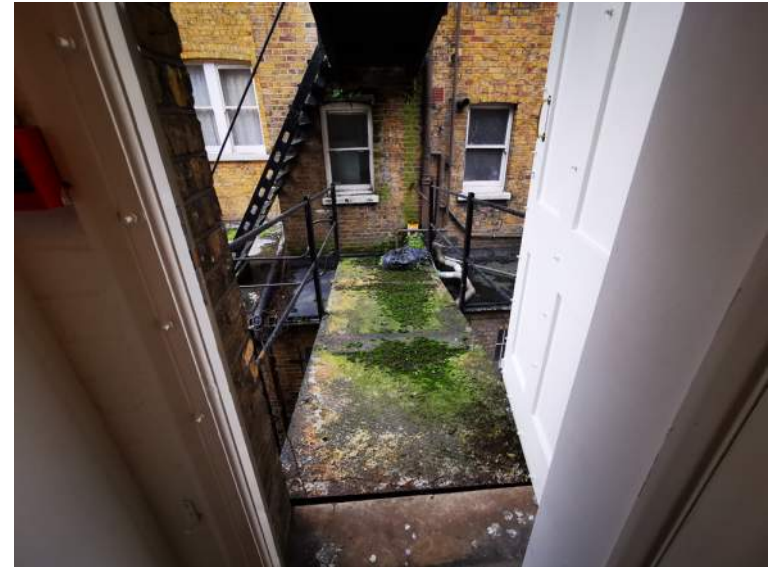
Fig. 21. dilapidated egress bridge poses safety risks
