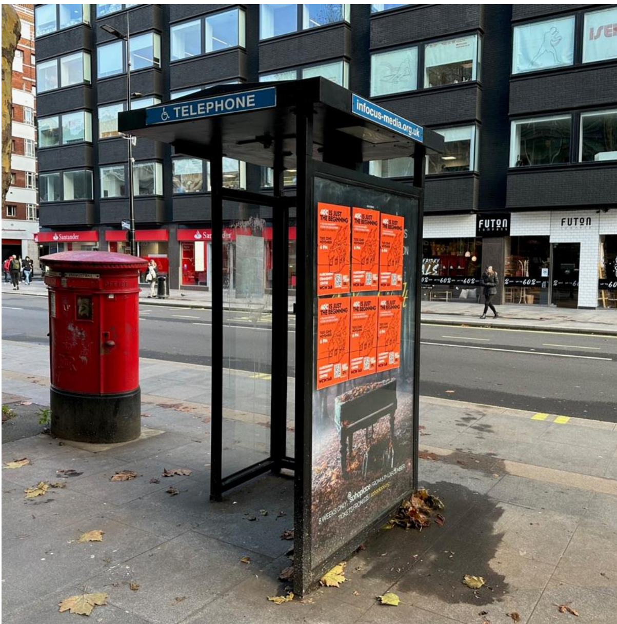
Site photograph taken 22 nd November 2022 showing fly posting and glue residue.
