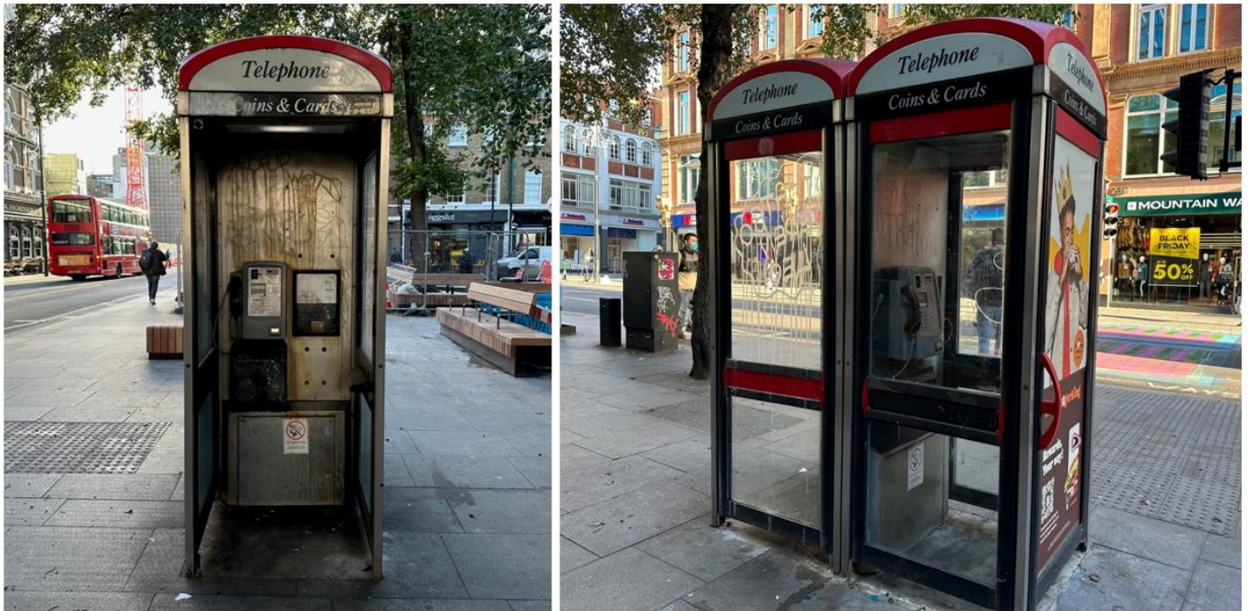
Site photograph taken 22 nd November 2022 showing the call box to be dirty and contain graffiti.
