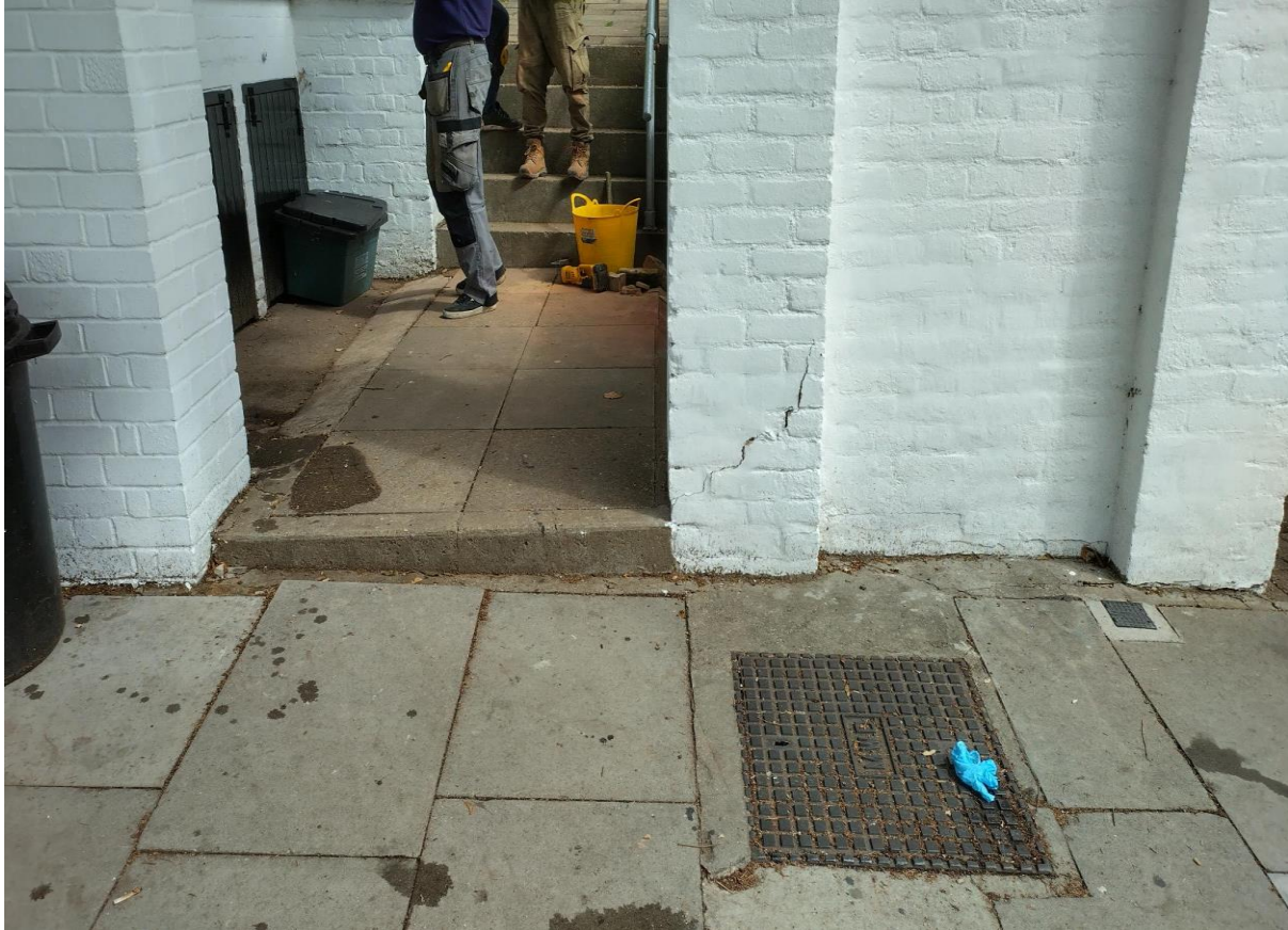
Photo 6 – Wall damage/gate pier (2)
