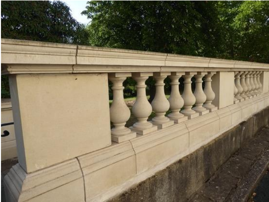
12.Cumberland Terrace: Reconstructed balustrade with obtrusive expansion joints
