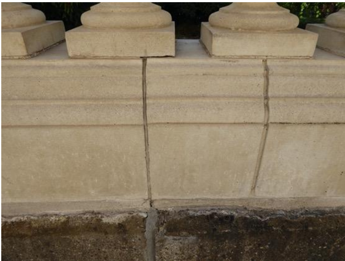
13.Cumberland Terrace: Obtrusive expansion joints in reconstructed plinth
