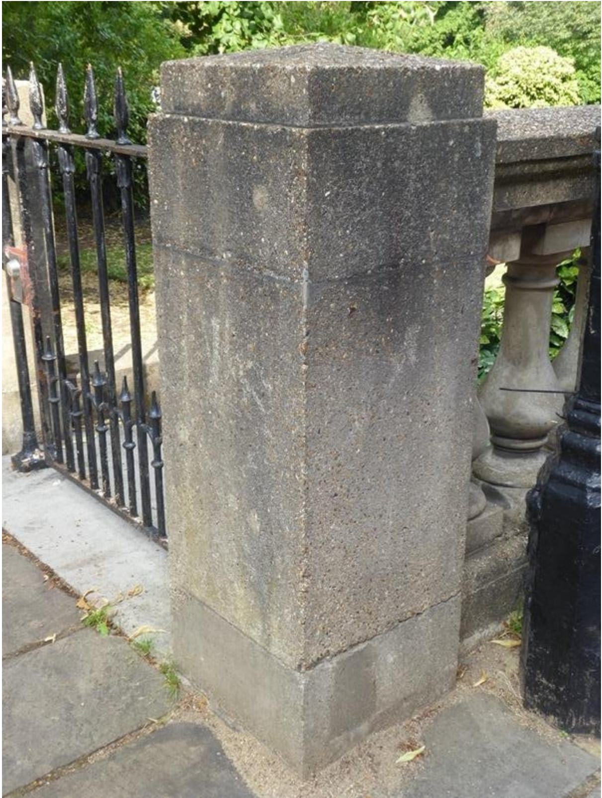
10. Pier showing aggregate finish and pyramidal cap with original cast iron gate to garden
