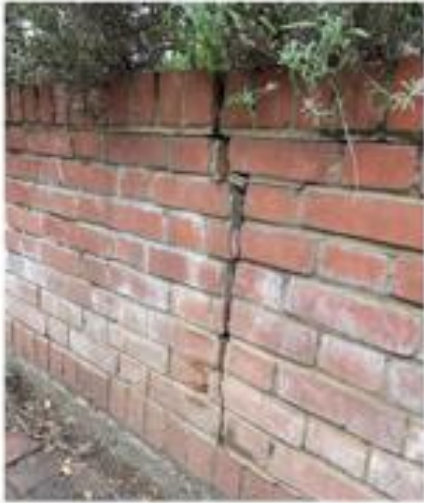
Photo 3 – Vertical tapering crack at approximately 2.4m from the tree towards the driveway
