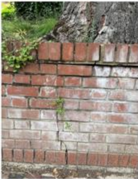
Photo 5 – Cracking at the tree location
