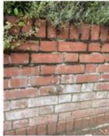
Photo 4 – Tapering vertical crack at about 2.3m the other side of the tree
