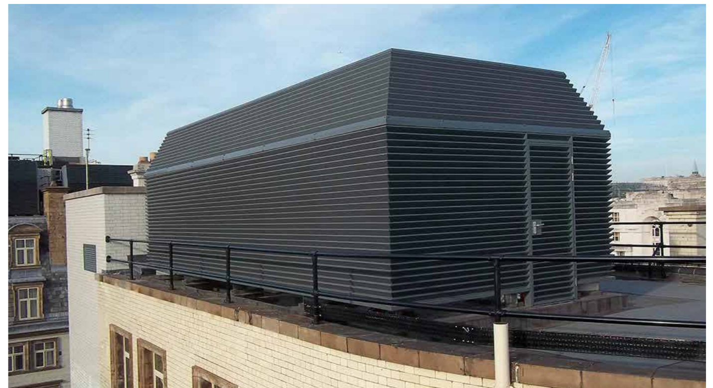
Example rooftop acoustic plant room
