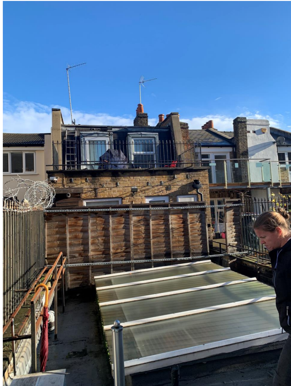
Existing Skylight To be replaced with new.
