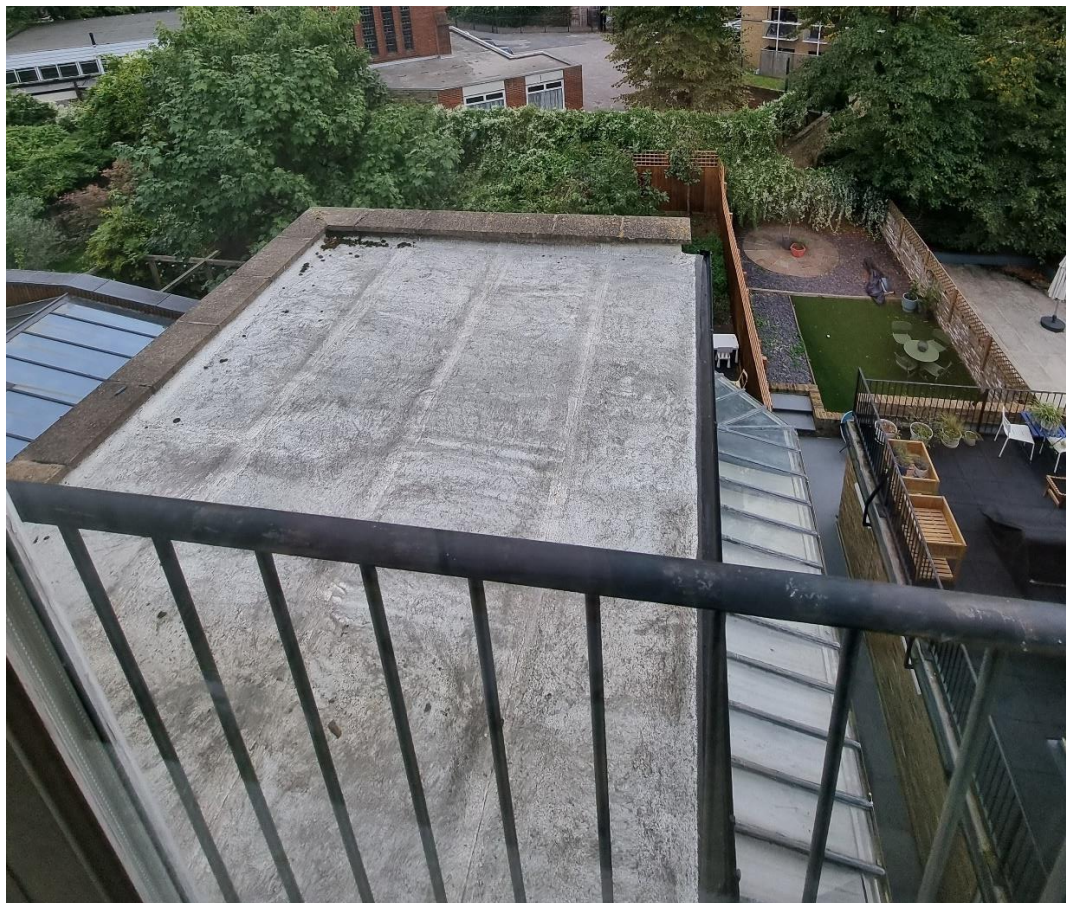
Figure 6. The existing closet wing roof with concrete coping. Note the existing first floor terrace to no. 25 to the right hand side © SEB + FIN Architects
