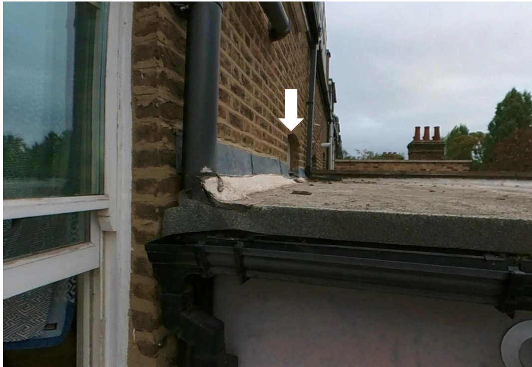
Figure 8. The remnant of the apparent stair landing window, with brick arch, looking north from outside the second floor study/bedroom. © SEB + FIN Architects
