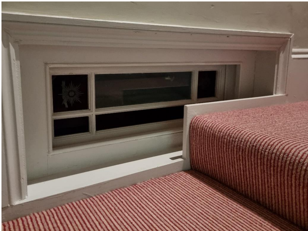
Figure 7. The remnants of what is believed to have been a large sash window to the rear stair landing (prior to the loft conversion and / or vertical extension of the closet wing). © SEB + FIN Architects
