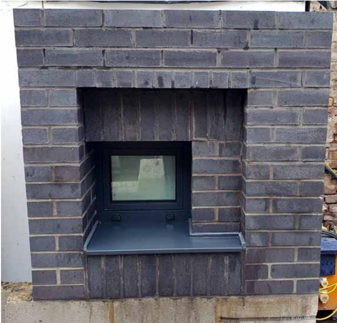
Sample panel 03 - illustrating White smooth facing brick. Dark coloured brick trim and panels are Black smooth brick, see sample panel 04 for manufacture reference.
