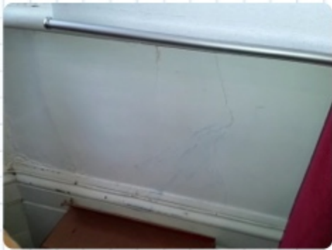
Crack below bay in living room
