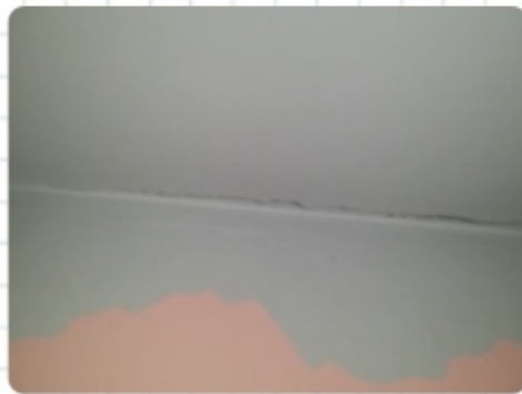
Bed 3-2mm Crack along ceiling
