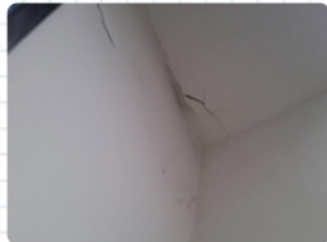
2nd floor hallway crack on ceiling
