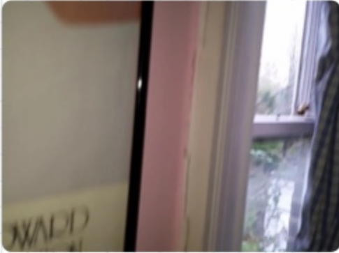
Separation crack between window and wall bed 3
