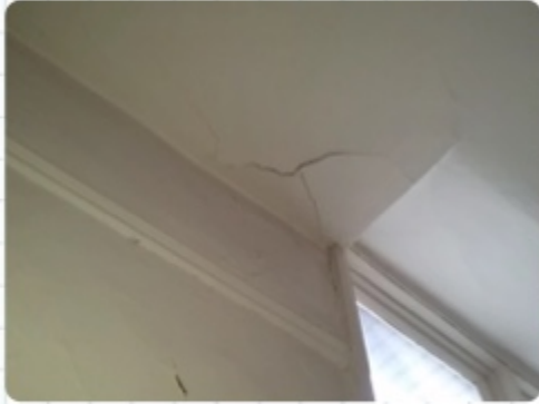
Crack in ceiling in dining room 3mm
