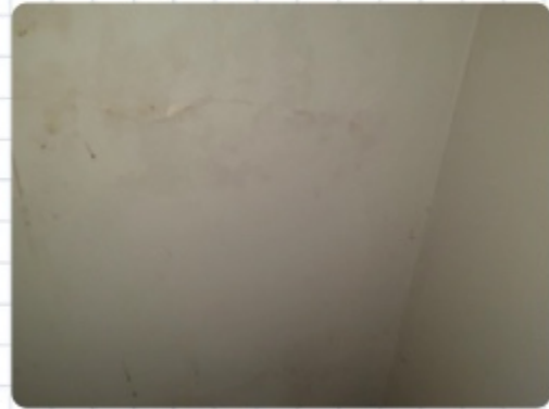
Hairline cracks on right of window in bathroom
