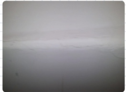
Crack in kitchen ceiling
