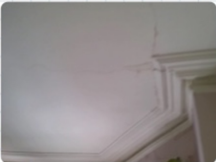
Crack on ceiling in master bedroom
