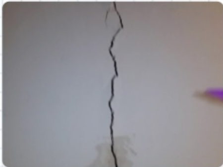
Crack on left wall of first floor hallway 10mm
