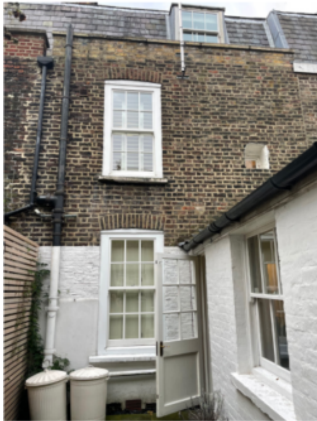
2. View of rear elevation and existing rear projection, boundary with no 16 to the left.
