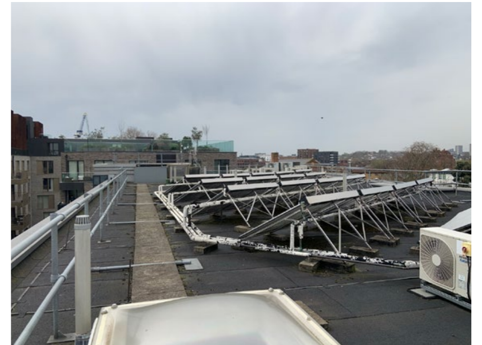
6. View of roof plant and solar panel located on the roof
