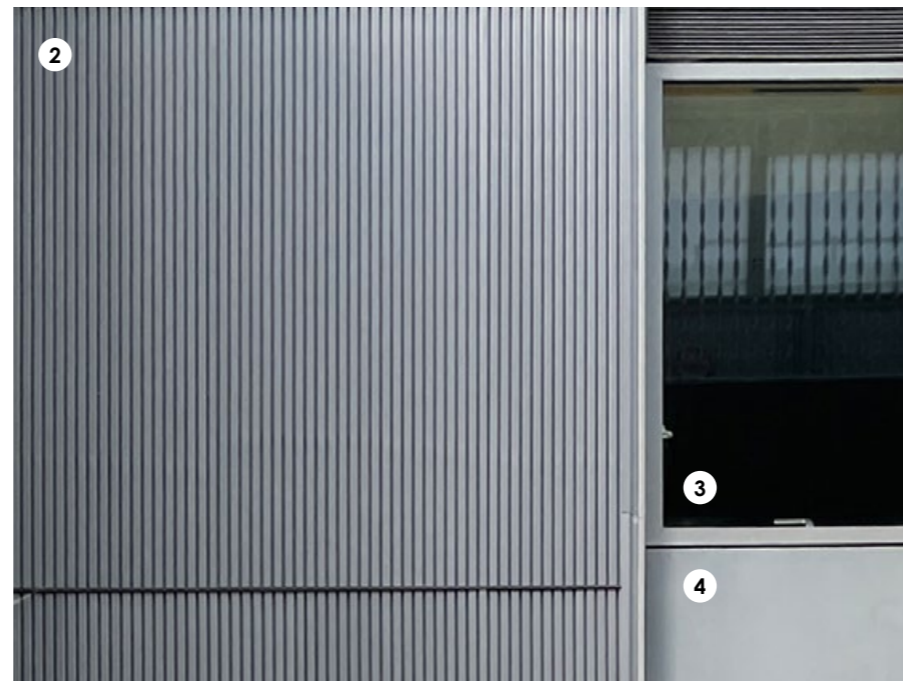
2. Fluted metallic cladding on the proposed fourth floor will match the existing floors below 3. Window frames and reveals to the proposed fourth floor will match those from the existing floors below 4. Flat panel cladding on the fourth floor will match the existing floors below
