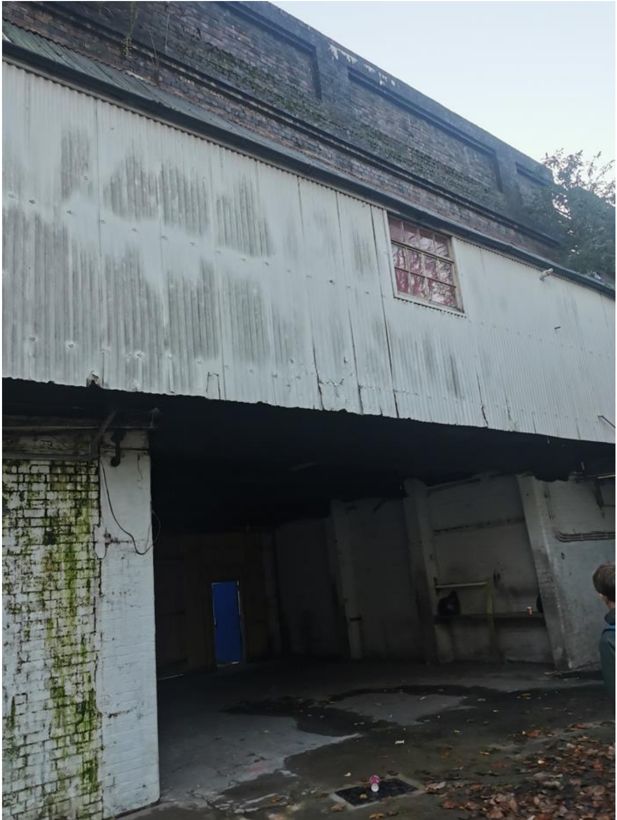
7. Unauthorised extensions in the yard area to be removed
