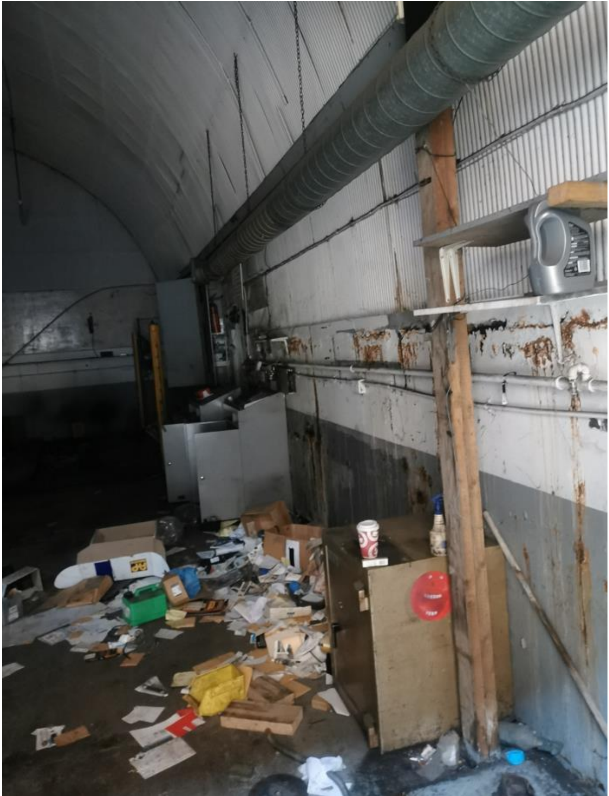
6. Derelict condition of many of the arches
