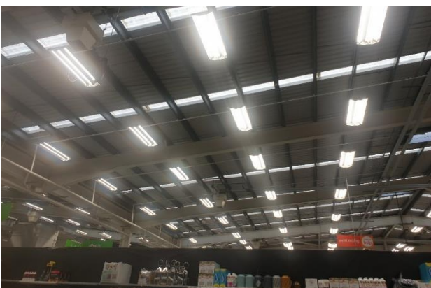
Figure 51 Main building WEEE lights (approximately 220 units)
