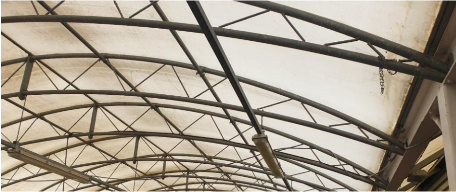
Figure 43 Garden area canopy – polycarbonate sheets
