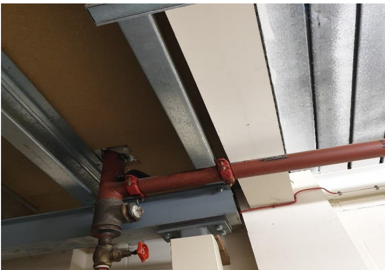
Figure 17 Transition between the composite floor and sales mezzanine with cold-formed joists (left)
