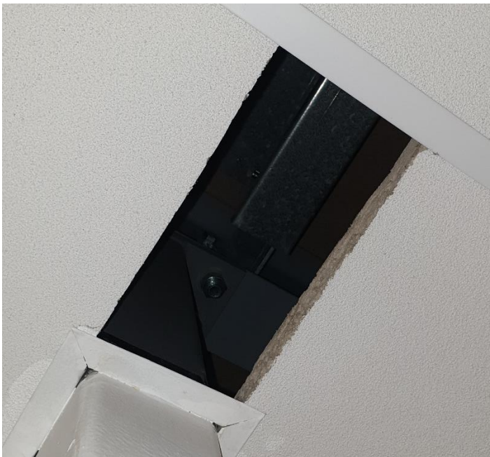
Figure 37 Sales mezzanine ceilings – opening found on site
