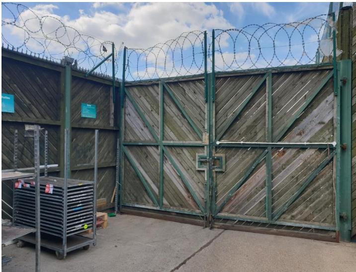
Figure 21 Posts, framing and razor wire fence
