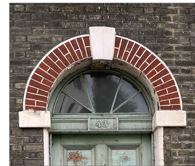
5 Adjoining House Door Scale: nts
