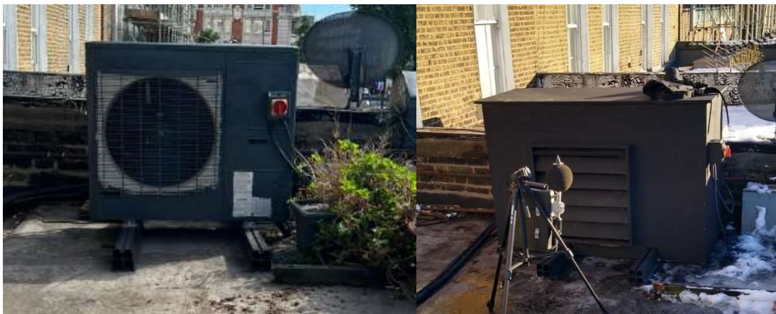
Figure 1.0 – AC Condenser without and with enclosure
