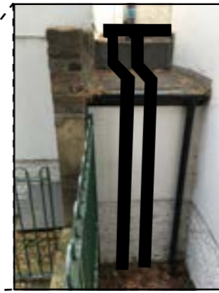
District heating pipework rise behind heating plant room B91. Refer to drawing UCL-BHE-00-00-DR-AM-2002
