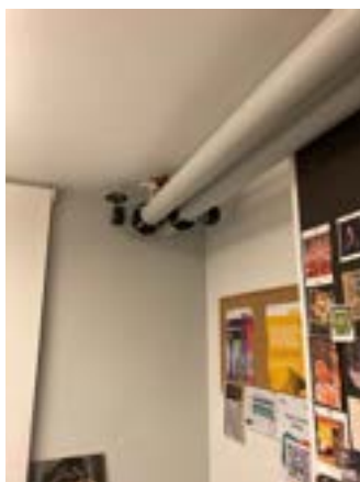
Figure 5: Pipework building entry point
