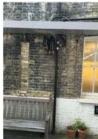
Figure 4; Pre-installed pipework flanges
