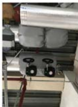
Figure 2: Existing DHN tapping point
