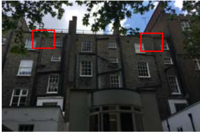
Existing Gas Boiler Flues
