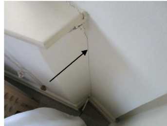
Cracking to left hand side of bay
