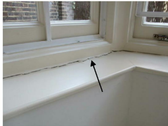
Cracking to bay
