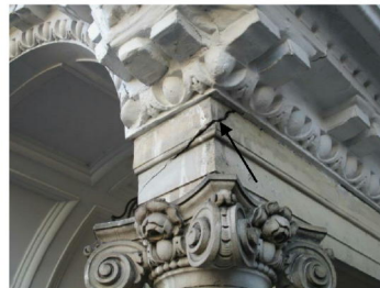
Cracking to portico
