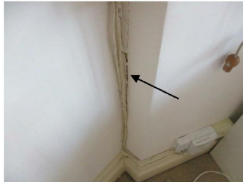
Cracking to right hand side of bay
