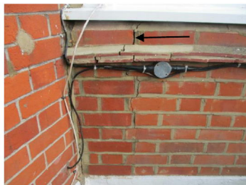
Cracking to bay
