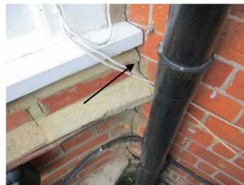
Cracking to bay
