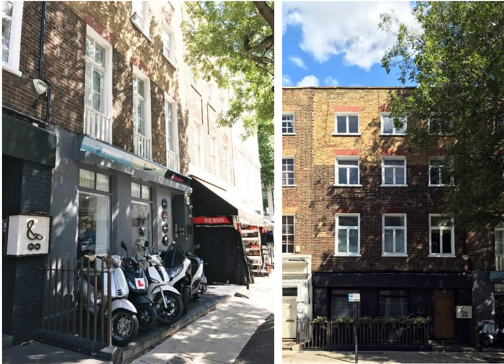
View of existing ground floor condition at 68 Charlotte Street and 70 Charlotte Street
