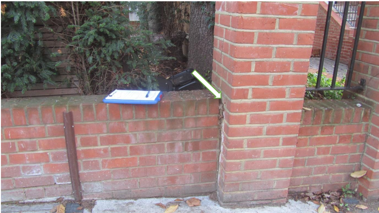
PHOTOGRAPH NO. 6 - BASE OF T1 ENCROACHING INTO THE CURTILAGE OF NO. 4, ALSO SHOWING MOVEMENT OF THE FRONT BOUNDARY WALL (ARROWED)
