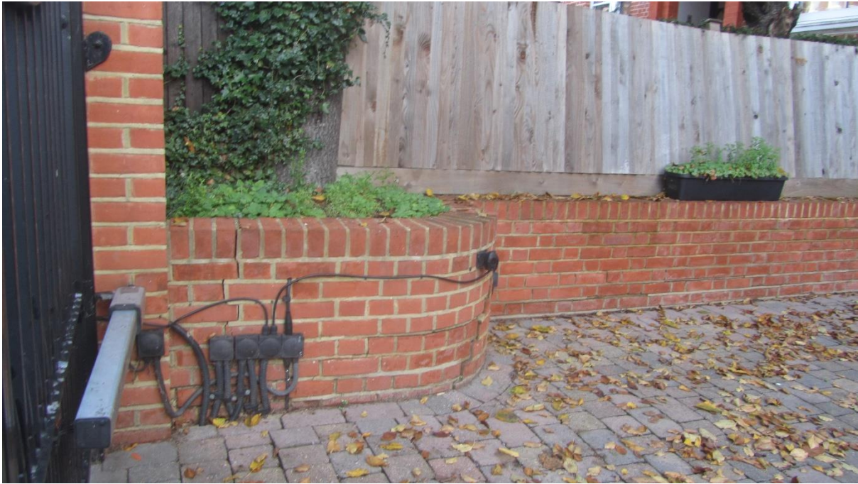
PHOTOGRAPH NO. 5 - CRACKING OF THE RETAINING WALL SOUTH OF THE TREE BASE
