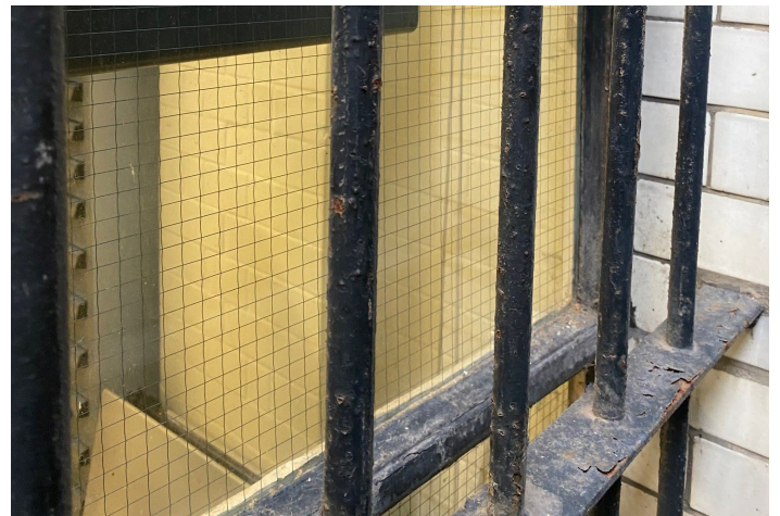
Photo corrosion of window frame at jamb.
