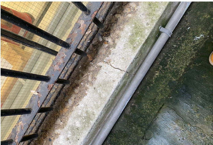
Photo of window showing corrosion of window frame and cracking of sill.
