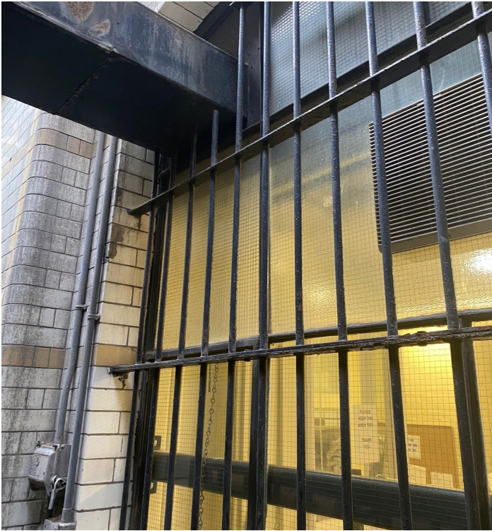
Photo of window showing redundant duct work and vents that may be removed on top left.
