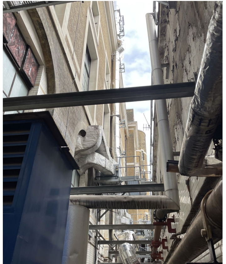
1. Photo of existing mechanical ducting on the south east elevation above the window
