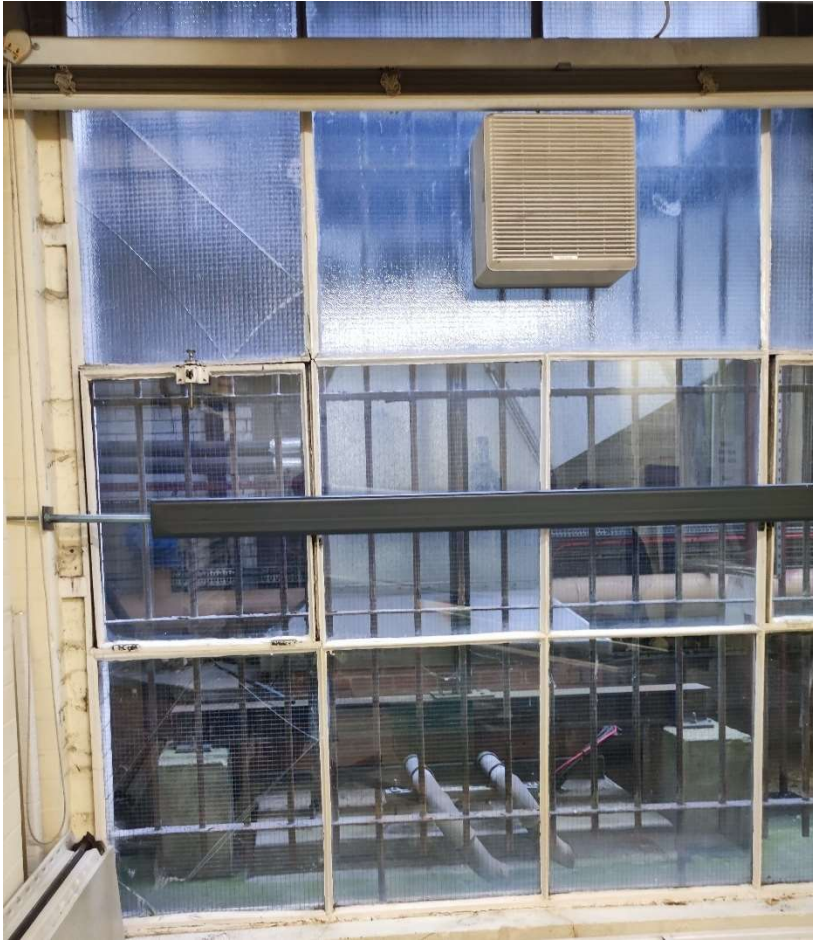
Figure 2: Expansion of window frame at base at east end and cracked window panes above
