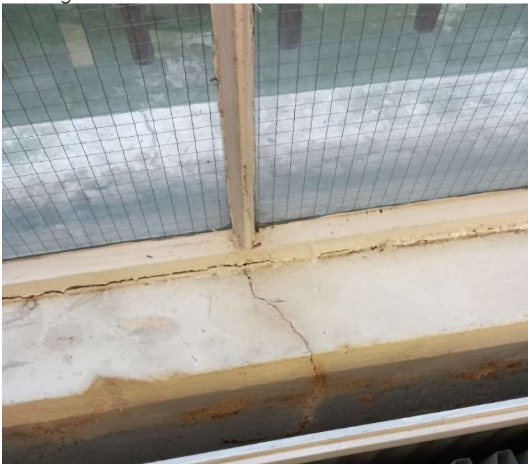
Figure 3: cracked window sill
