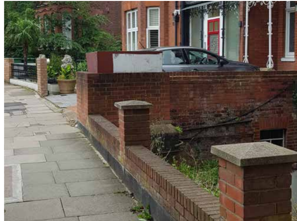
FIG. FRONT LIGHTWELL BOUNDARY WALL - IMAGE 02
