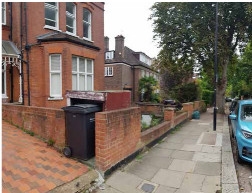
FIG. FRONT LIGHTWELL BOUNDARY WALL - IMAGE 03
