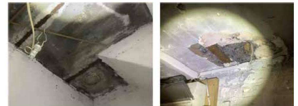
CORRODED STEEL BELOW DRIVEWAY SEEN FROM BELOW
