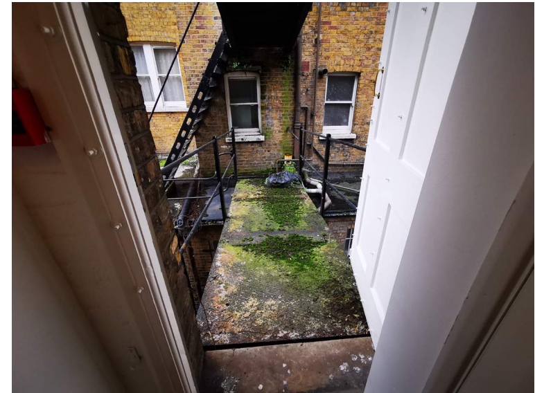
Fig. 21. dilapidated egress bridge poses safety risks
