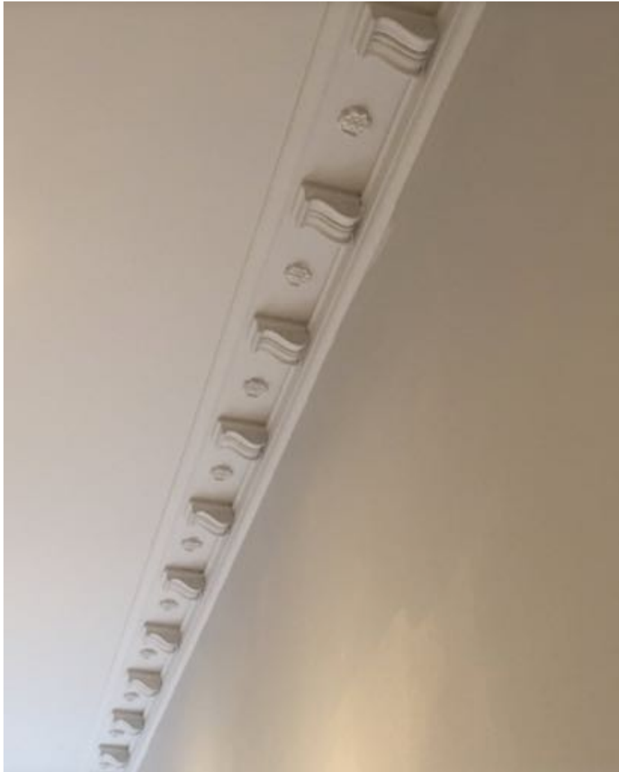
Cornice LV414 with Blocks and Rosettes
