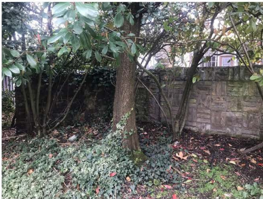
Plate 3: Photograph of the boundary wall from the garden. Note: the map regression provides evidence of alterations to the walls in the garden through the addition of a curved element which has since been partially demolished.
