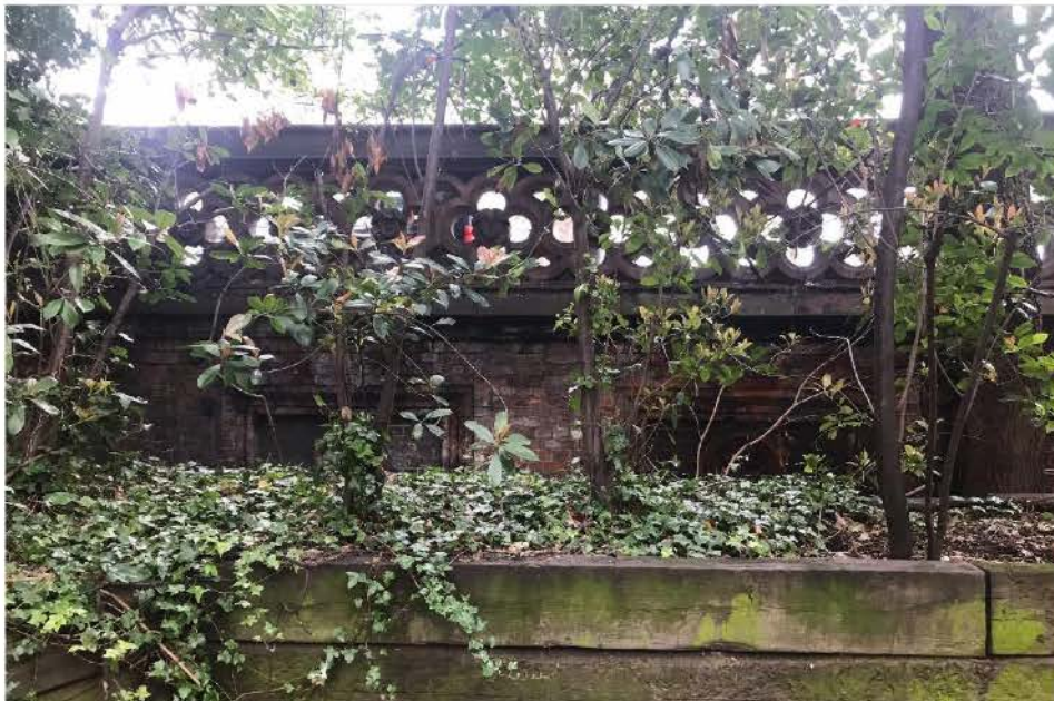
Plate 6: Photograph of the Grade II listed bridge forming the western boundary of the site from within the garden of 2 Park Village East. Note that this part of the garden suffers from recurrent fly tipping from the bridge and has led to the accumulation of rubbish.
