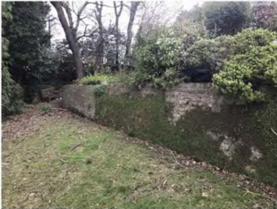
Plate 7: Photograph of the multi-phase retaining brick wall dividing the two principal levels in the garden. Note: the end section of this wall is evidently more modern than the central moss covered section and was likely added when the curved connecting wall was partially demolished.
