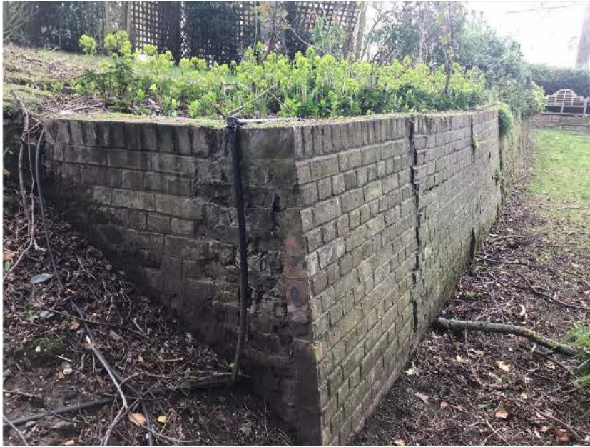
Plate 5: Photograph of the brick retaining wall which divides the two principal levels within the garden. Note: this wall is evidently multi-phase and is made up of historic and more modern brickwork. This end of the wall was likely added when the late 19 th century curved wall was partially demolished. Overall the retaining wall is in a relatively poor condition and is suffering from leaning and excessive cracking in places.
