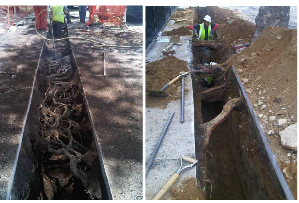
Airspade trench reference images. Display principles of method only. Excavation to be no wider than 400mm and no deeper than 450mm.
