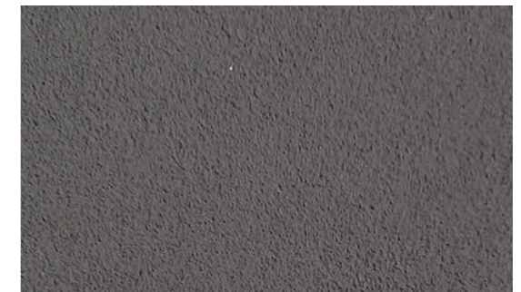
4. Existing render to the facade painted dark grey
