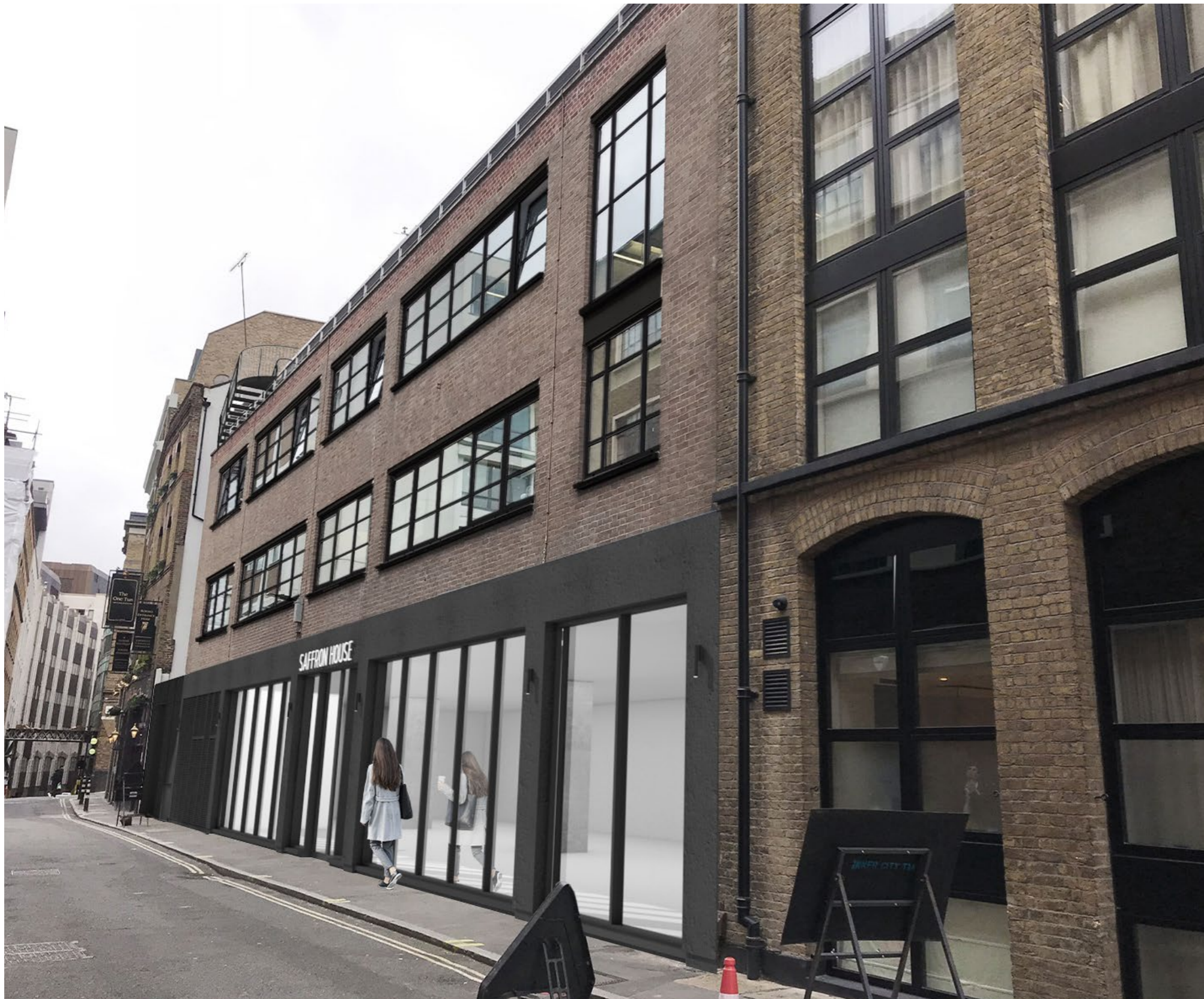
Far right opening is widened and door replaced with window. Window/door frames replaced and render repainted at lower ground floor. Window frames at upper ground floor and first floor repainted to match.
