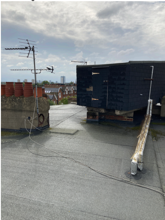
Further view of tank room
