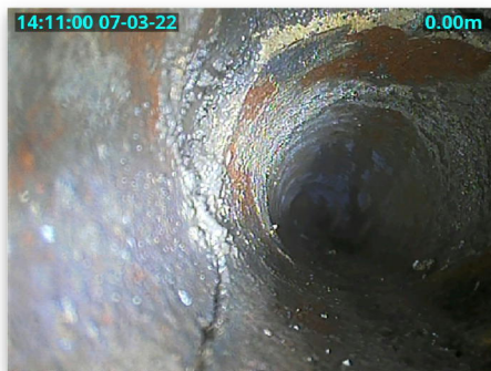
Fig 3.3 :Cracked Gully Base
