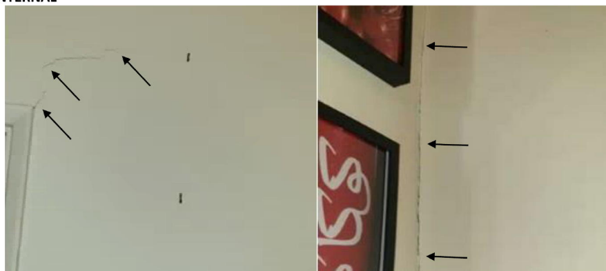
Tapered cracking above door frame
