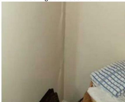
Cracks underneath lining paper.
