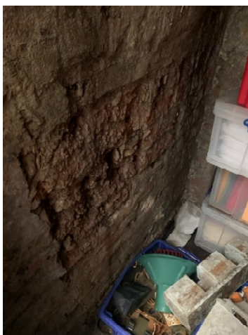
Images showing brick erosion
