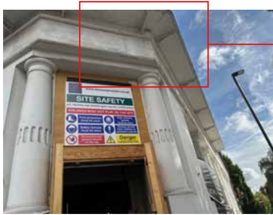
Existing damaged plywood panel on fascia
