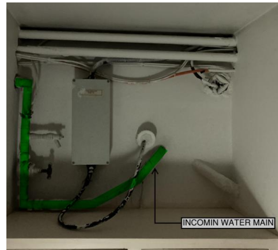
Figure 4 – Jockey's Fields Side Lead Water Main
