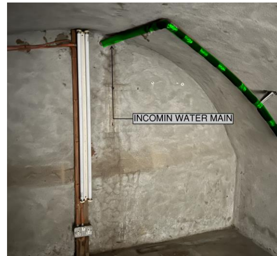
Figure 3 – Bedford Row Side Water Main
