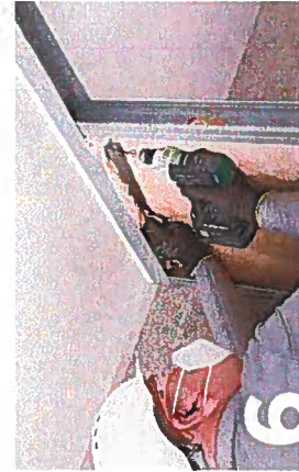
6 Add appropriate ISOVER insulation (Acoustic Partition Cell (200) as shown) within the partition cavity to contribute to acoustic and thermal performance where required.
