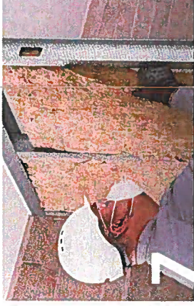
7 Stone mineral wool (or other) may be required as part of the partition installation, particularly for situations requiring enhanced fire resistance.
