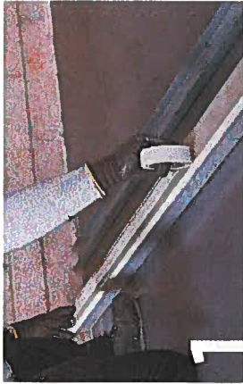
1 If a deflection head is required start by creating the correct width of the deflection head and width of Gyproc clasterboard or Glasroc spec. list board and attach to your head and wall. Use appropriate Gyproc FireStrip as per the detail.
