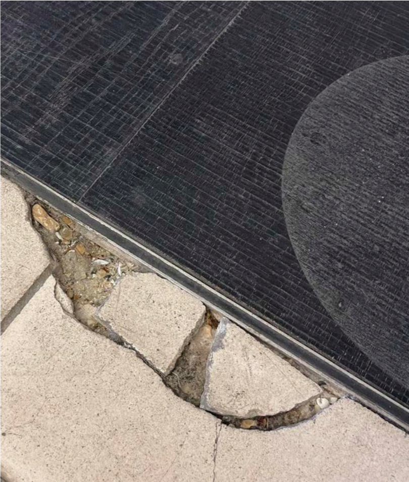
Existing tiled flooring is cracked in places.
