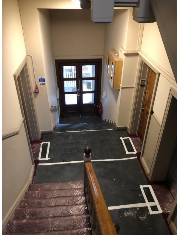
Fig 2 - No 10A South Square Internal flight of stairs from front door to raised ground floor
