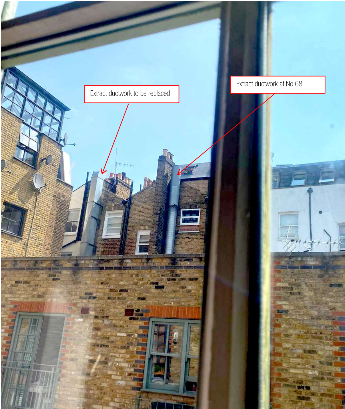
Photo of the rear elevation showing the existing ductwork to be replaced
