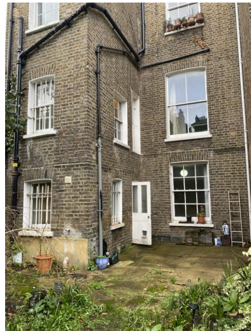
Figure 27: Rear elevation with windows and doors to outrigger. This shows the redundant doorway that disrupts the composition of the rear elevation.
