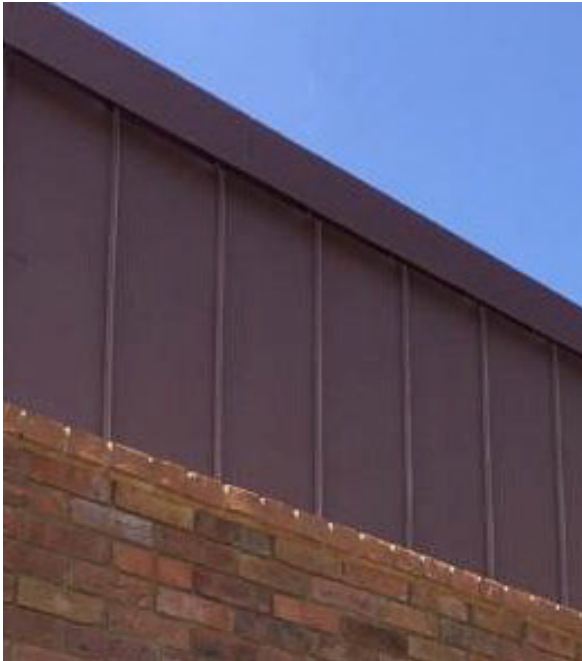
Image of the red pigmented standing seam zinc cladding proposed for use on the plant screens.
